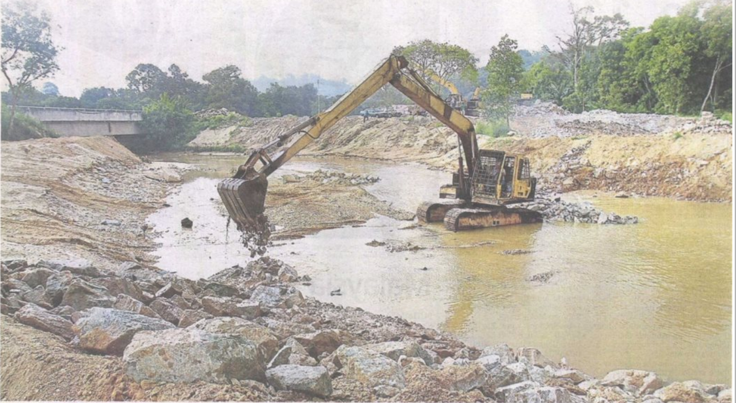
Mitigation works: A worker on an excavator expanding the banks of a river in Rawang, Kuala Lumpur, to prevent flooding whenever it rains. — FAIHAN GHANI/ The Star
